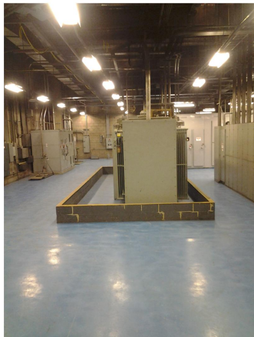
TRANSFORMER & SWITCHGEAR INSIDE EXISTING CONTAINMENT SYSTEM
