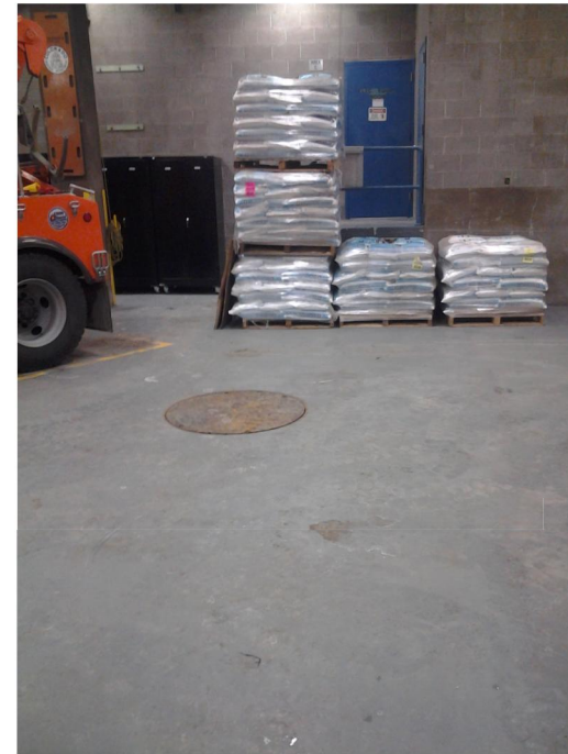
OUTER GARAGE BAY MANHOLE LID ABOVE WASTEWATER SAND FILTER BEDS
