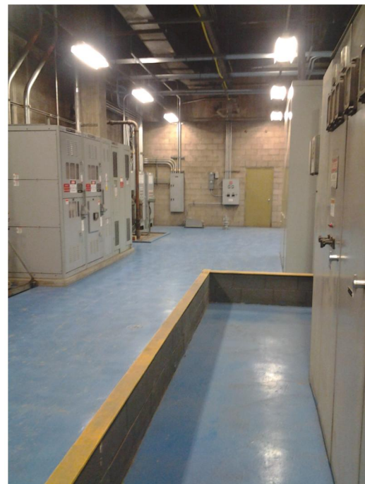
TRANSFORMER & SWITCHGEAR INSIDE EXISTING CONTAINMENT SYSTEM
